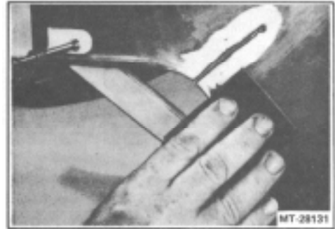
Figure 33. - Sanding Exterior Damaged Surface (Crack Shown - Typical)
